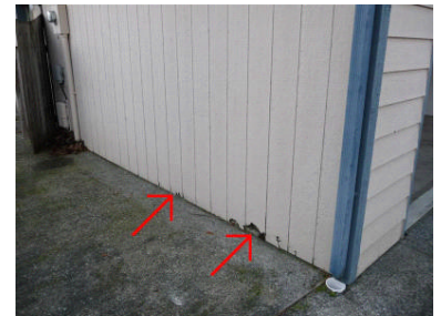
Siding is water damaged
